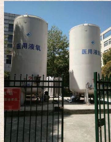
The Hospital's liquid oxygen storage tanks
